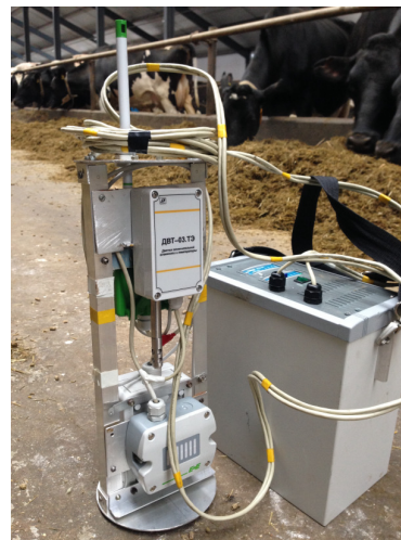
Fig. 2. Portable installation for inside climate monitoring
